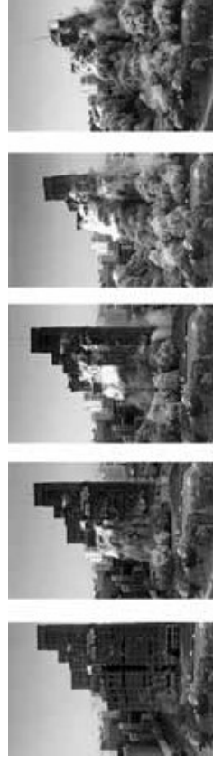
Figures 5: Demolition of Hudson's department store in 1998. (Source: image sequency by Lowell Bolleau).
